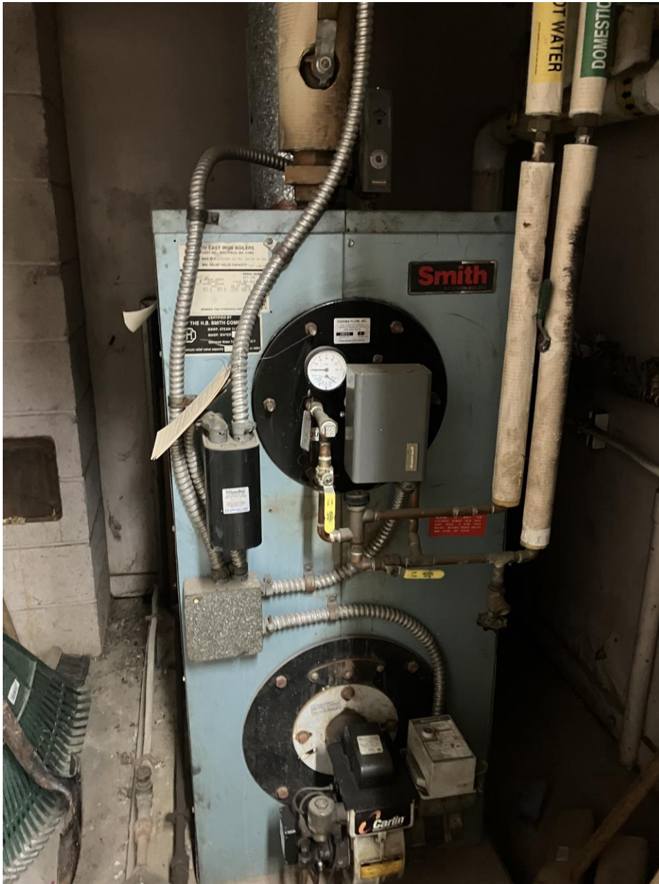
4- Smith Boiler in Basement of Main Building
