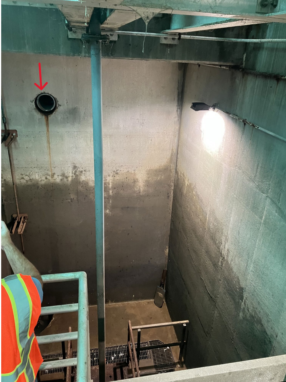
3- Main Pump Station Overflow Pipe Noted
